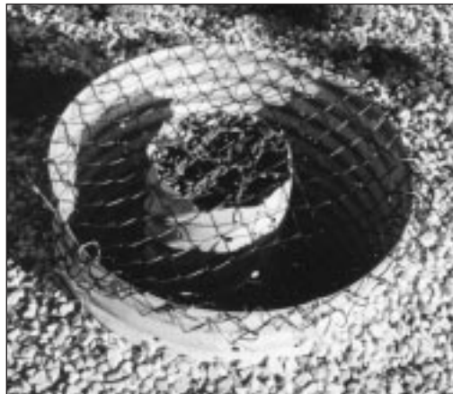
Stormwater outlet designed to reduce sediment discharge
