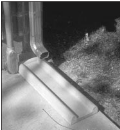
Downspout disconnect and redirected to ground
