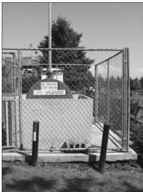
Containment dike to contain accidental spills from above ground tanks
