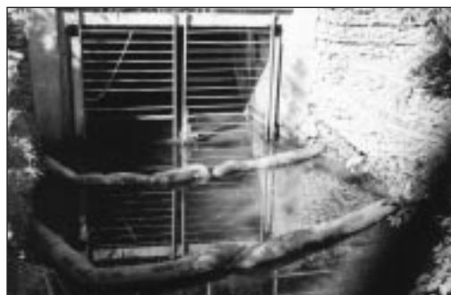
Oil booms like these on a storm sewer wouldn't be necessary if used oil recycling programs were in place
