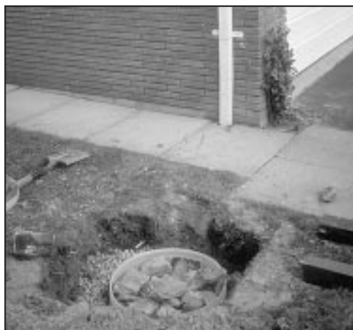
Soak-away pit for downspout disconnect
